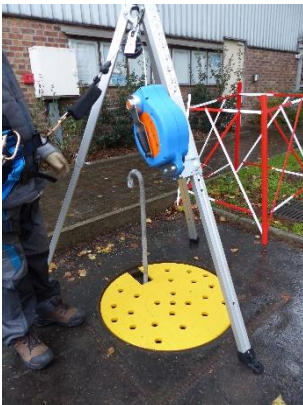
Manhole cover with anchor rod
